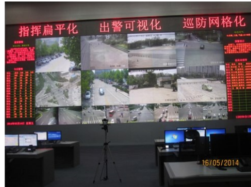
Command Centre in Weifang City
